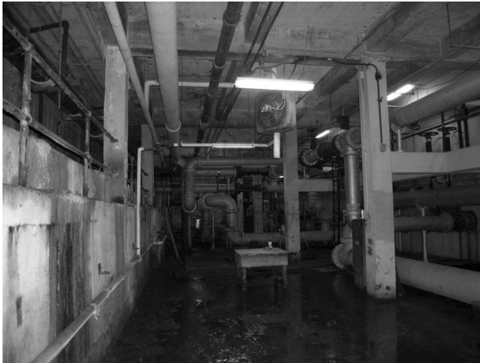
Figure 10 Pump room, Astoria Park Pool and Bathhouse, Queens, New York City, view of the pipes that deliver water to and from the raised filter beds (on the right); the heating system has been dismantled. Photographed in 2006
