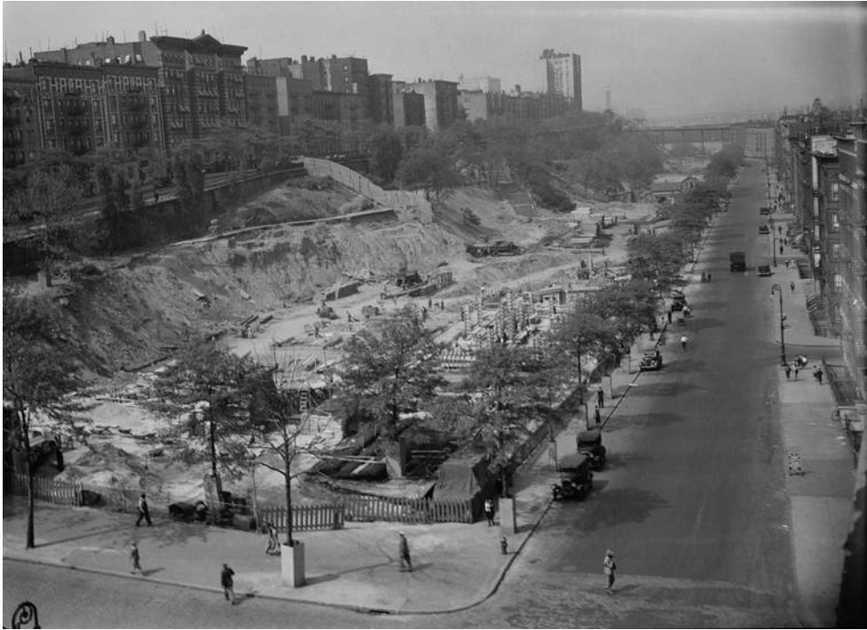
Figure 11 Colonial Park Pool and Bathhouse, Central Harlem, New York City, view of construction, 13 May 1936
