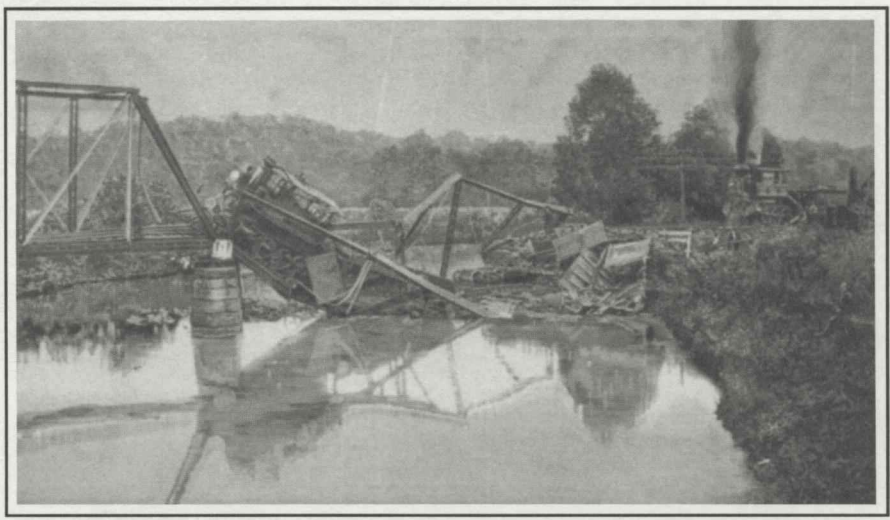
Fig. 10 —When a B&O locomotive hit a cow on this pin-connected bridge on April 30, 1887, throwing her into the truss, the bridge collapsed.
