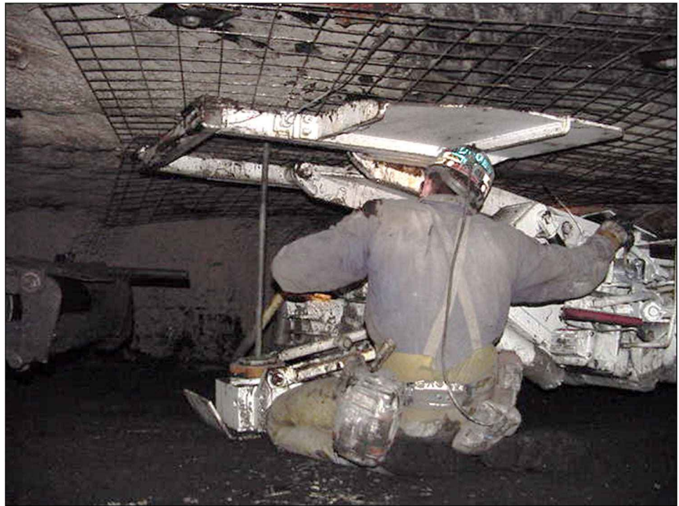
Fig. 11 Installing a roof bolt with screen in a low coal mine (photo by the author)
