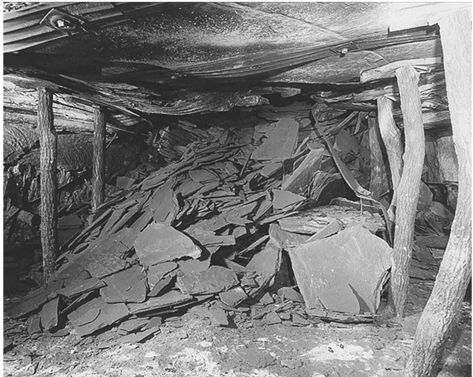
Fig. 3 A large roof fall in ground that had been supported by roof bolts and wood posts. McCormick (1969) estimated that 500 large roof falls occurred for each one that caused a fatality (source: US Bureau of Mines)
